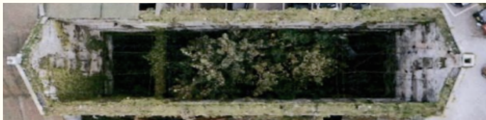
Aerial view of the roofless mill building, visibly no floors remaining just foliage growing throughout.
